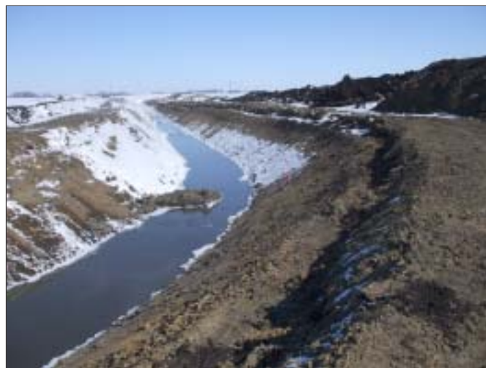
Work on Drainage District 65 continued through the difficult winter. Redings Gravel and Excavating of Algona was the contractor.
