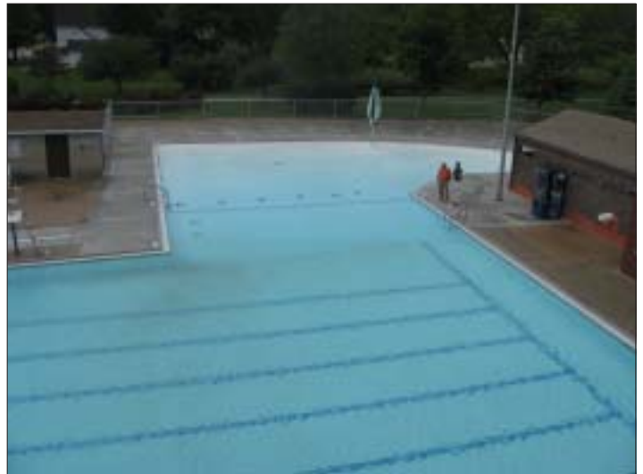
Looking out at the new 2,300 square foot zero depth addition to the swimming pool in Belmond are Earl Zimmerman (left) and Kent Brcka, of Henkeo Construction. The bathhouse in the right of the picture was renovated in 1994 to a design completed by KPL. The picture was taken from atop the new 20 foot high slide.
