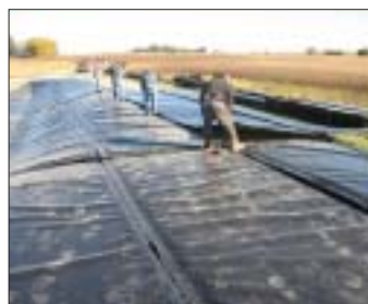
Covering the lagoon at the Strawberry Point Wastewater Facility.
