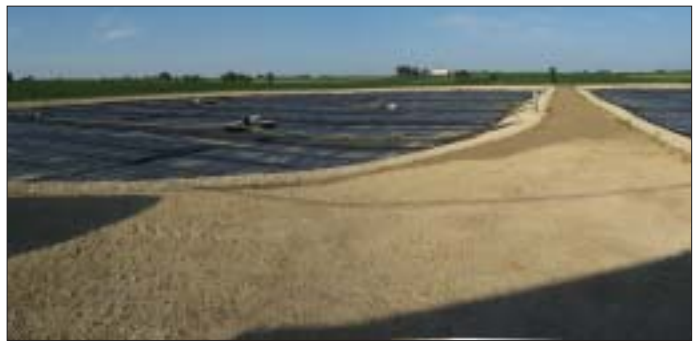
New lagoon at Strawberry Point. This project is producing effluent with less than 10mg/l CBOD and TSS and less than 1mg/l ammonia nitrogen.
