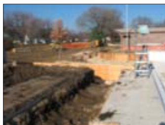
Construction of the zero depth addition to the Belmond pool. This photo was taken November 19.
