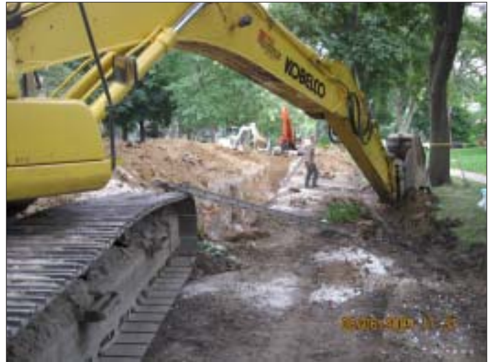
Construction on 10th Avenue in Fort Dodge, part of a 13 block street improvement project.
