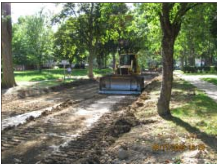
Construction on Phase One of a 13 block street improvement project in Fort Dodge is underway.
